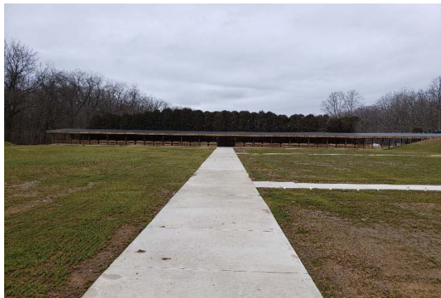
View of new shooting line for 100-yard range prior to baffle construction
