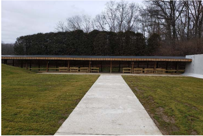
View of new shooting line for 50-yard range prior to baffle construction
