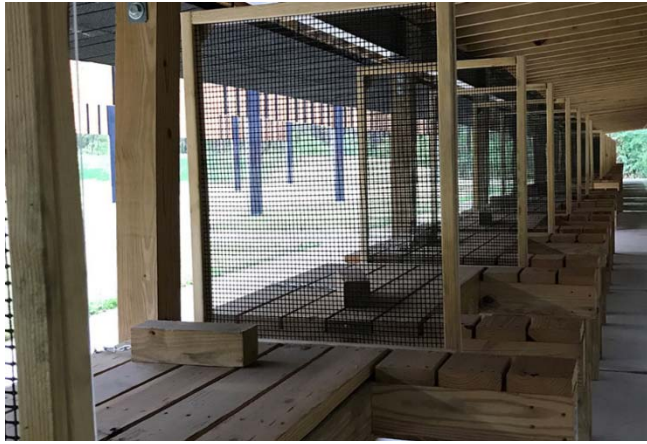
Continuous shooting line for 25-, 50-, and 100-yard ranges with newly constructed benches and social distancing barriers
